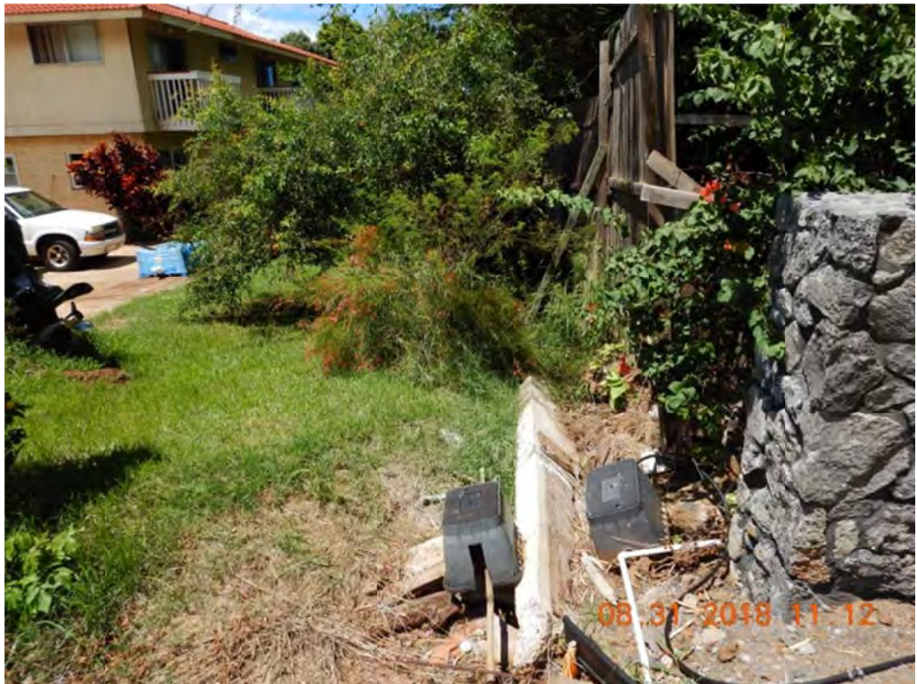
Photo 6: Existing swale appears to be created by flood water. Location is at north of DI shown in Photo 5.
