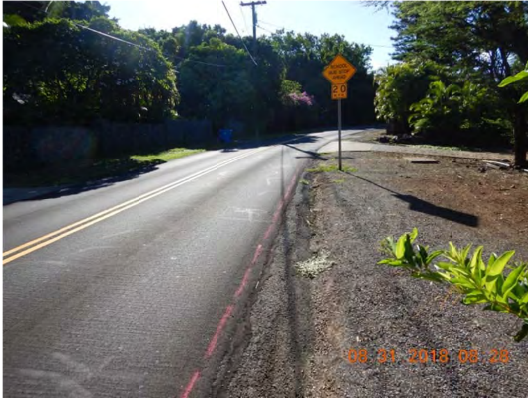
Photo 1: Stand on Mapu Pl, look mauka toward the driveway at Private property 2-1-015: 048 (fading ac swale)
