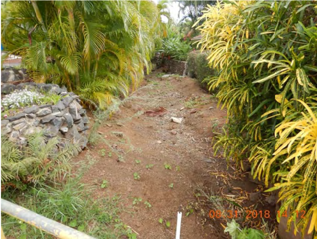
Photo 5: Stand on Kumulani Dr by the DI shown in Photos 3 and 4, Look toward downstream of the DI.
