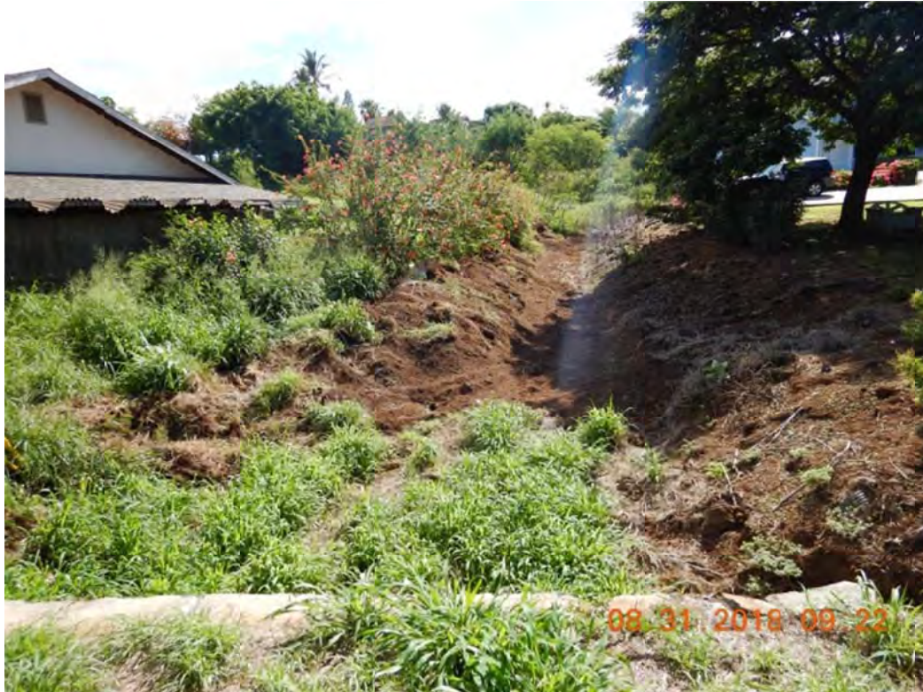
Photo 1: Stand on Mapu Pl, look toward upstream of Culvert 32, dredged materials were left on site.
