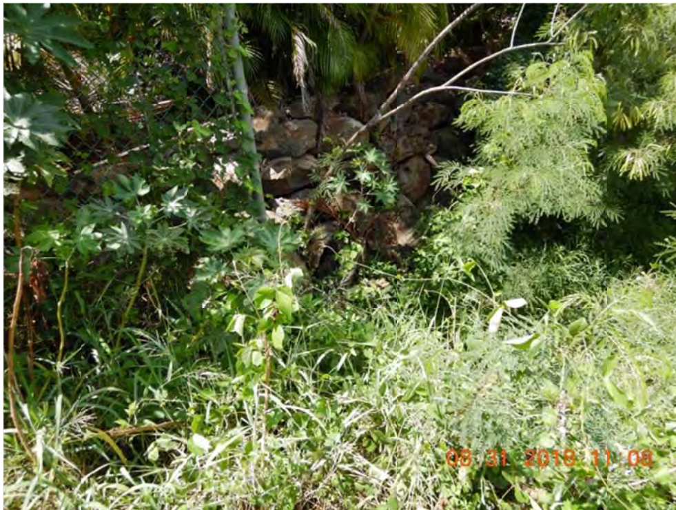
Photo 4: Close-up view of downstream channel at Culvert 43 outlet. Heavy vegetation was observed.
