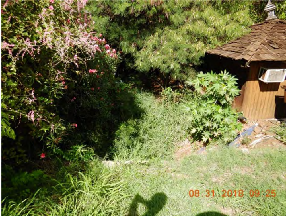
Photo 5: Stand on Mapu Pl, look toward downstream of Culvert 32 heavy vegetation was observed
