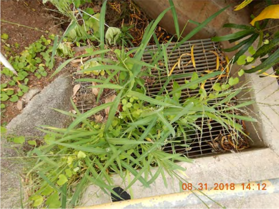
Photo 4: Close-up view of DI shown in Photo 3
