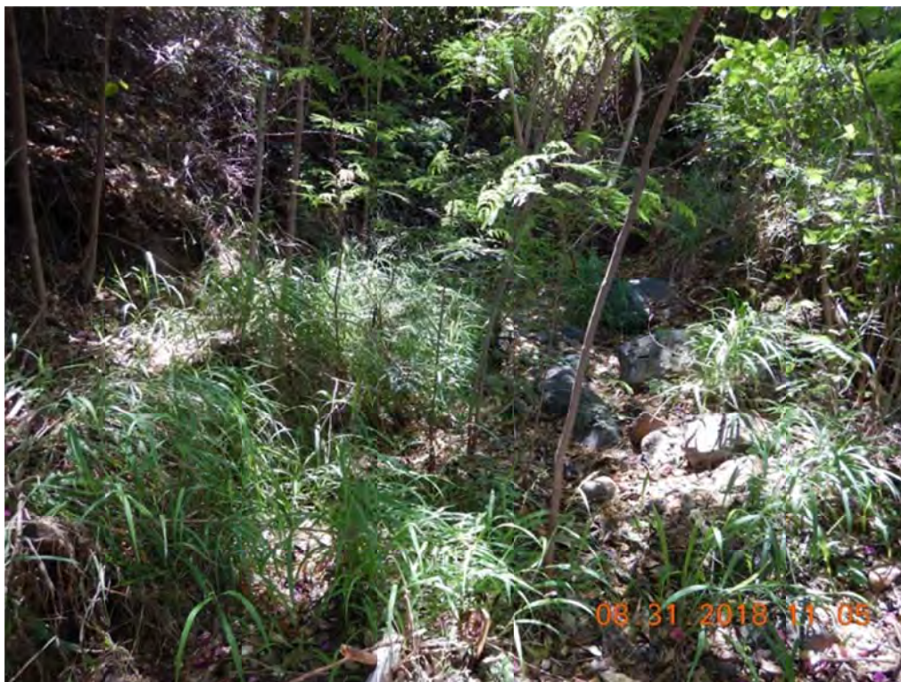
Photo 2: Stand on stream by Photo 1, look toward upstream channel of Culvert 43. Heavy vegetation was observed.
