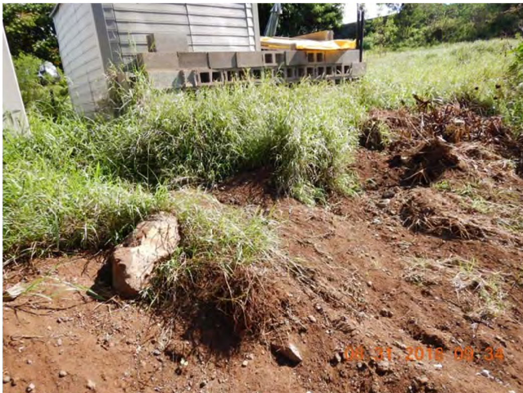
Photo 2: Further upstream of Photo 1, erosion was observed at the bank by the private property, TMK:2-1-015: 061.
