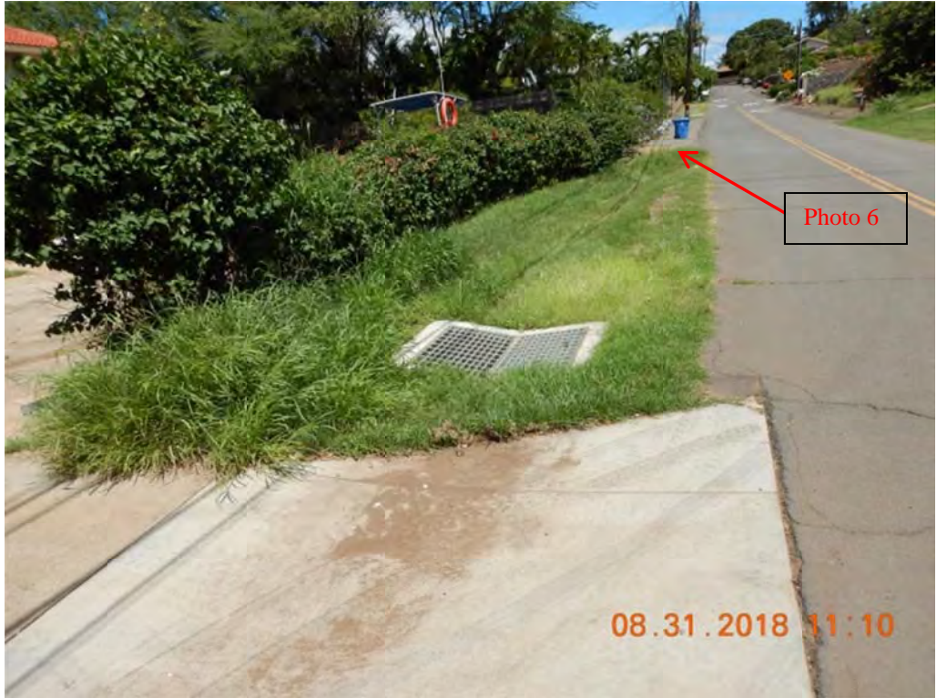
Photo 5: Roadside swale and drain inlet by private property TMK: 2-1-014: 087
